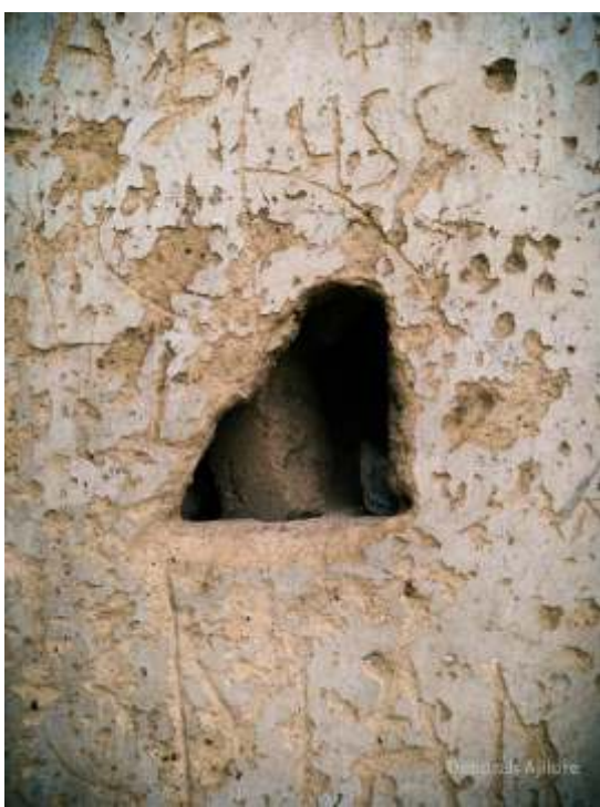
The Damaged Wall Ajilore Deborah Photography, 46x61cm
